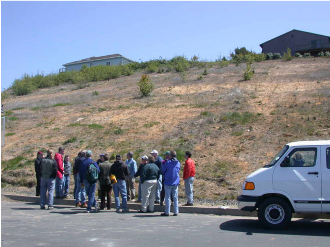
Figure 3: Parking lot behind Newport Middle School. This slope was cut to extend parking and road access. It contains paleodune deposits overlying weathered mudstone. The initial grades were too steep, resulting in gullying and small slumps in the paleodune deposits after winter rains. The paleosol near the middle of the slope reduced drainage and lead to excess surface runoff causing gullying of the weakly cemented paleodune sand. The slope has been mitigated by installation of geotextile nets and grass seeding, and a lateral drainage system. Photo from Peterson et al. (2003).
