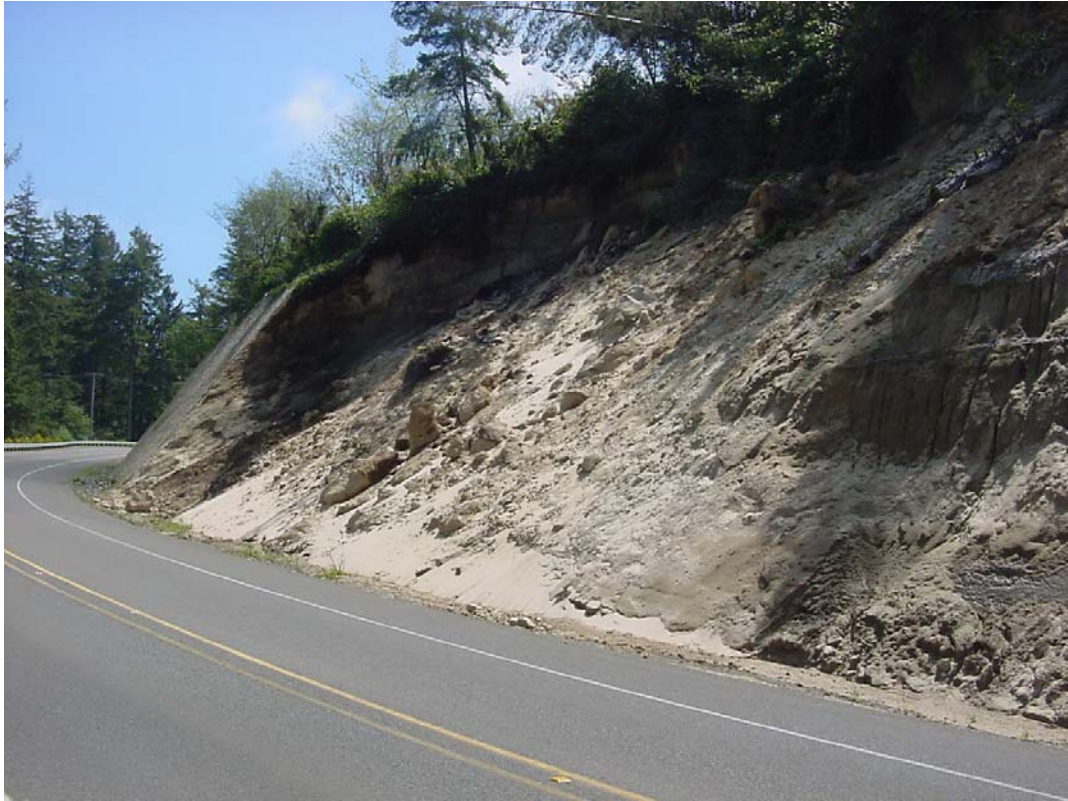
Figure 46: Large road cut failure along Canary Road south of Florence. Slope was cut at 57^{\circ} to widen the road shoulders.
