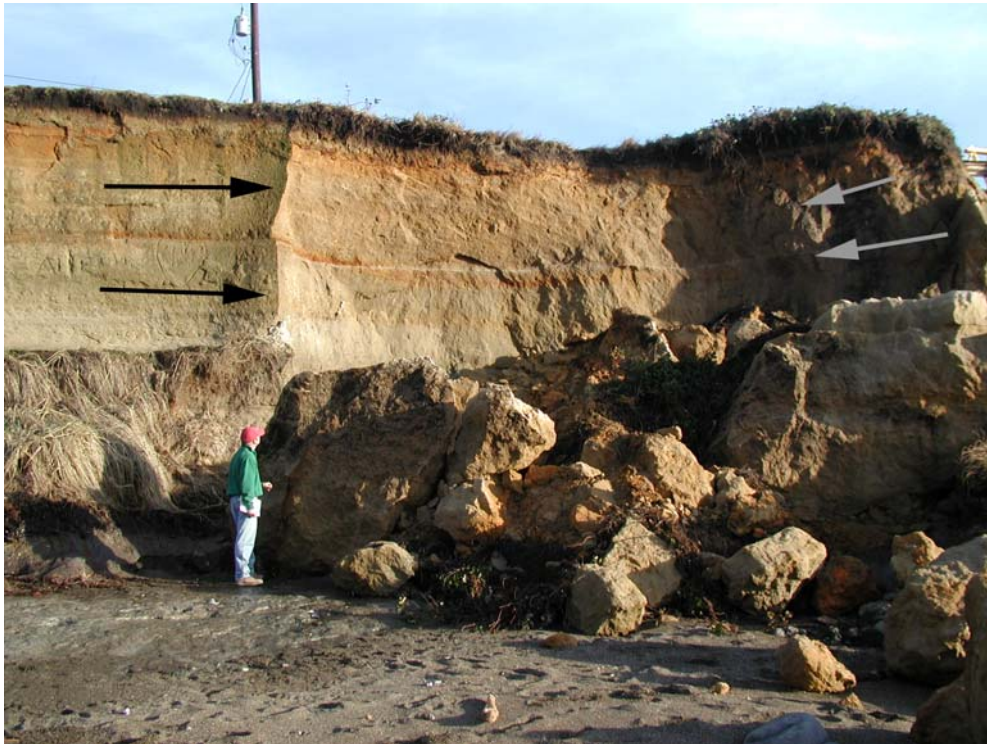
Figure 36: Sea cliff failure in Yachats located a few meters from a city street. Block failure occurred during a winter storm event in 2004. The failure may have been the result of ocean wave undercutting the sea cliff.
