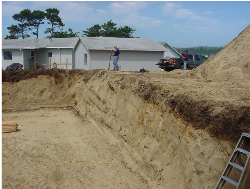
Figure 25: House foundation excavation situated on a paleodune deposit located on top of a sea cliff at Ona Beach.
