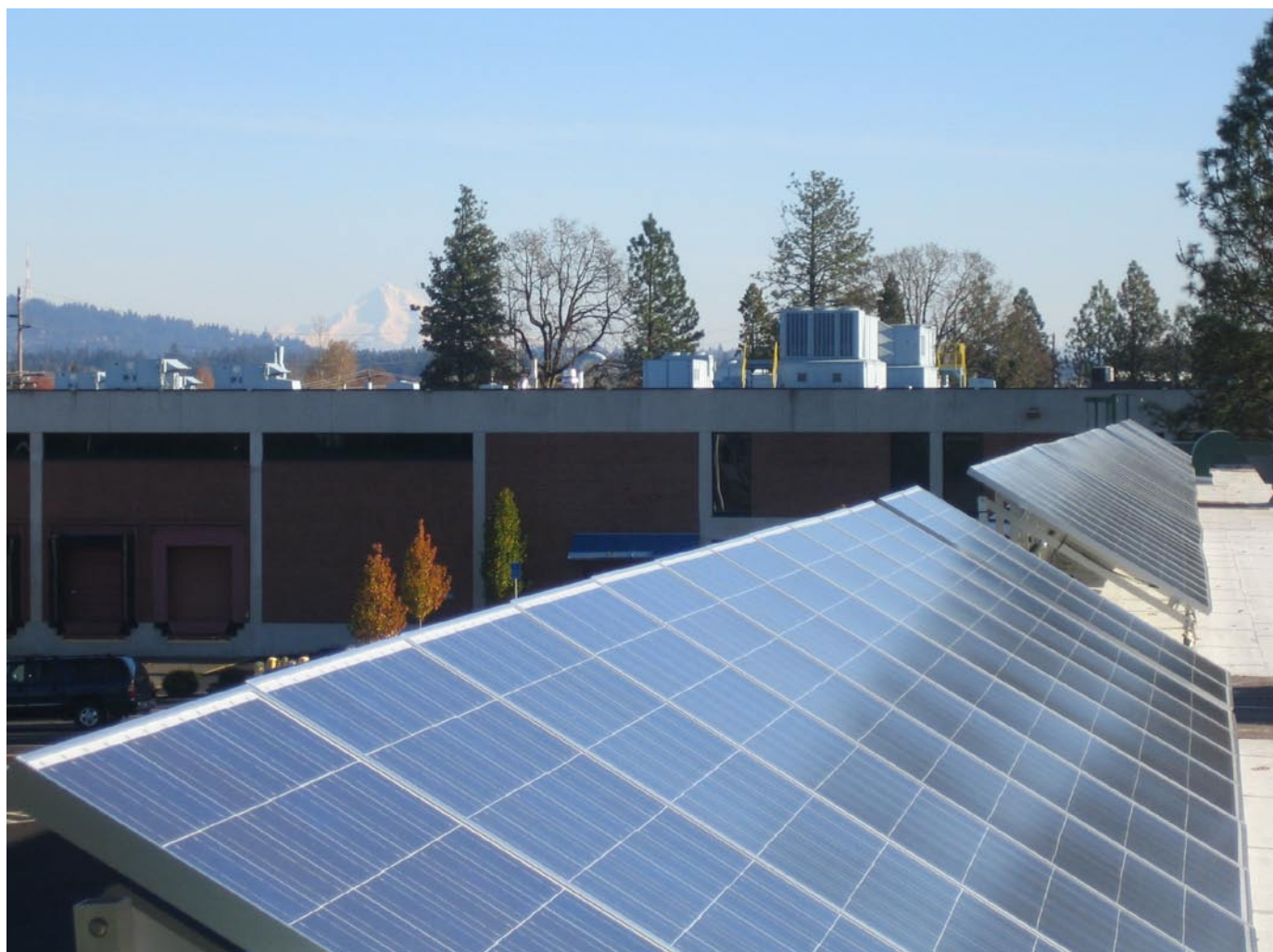
View of the roof panels that made up Phase 1. In the background is Mt. Hood.
