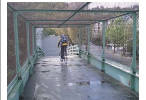
Water ponding on bridge surface
