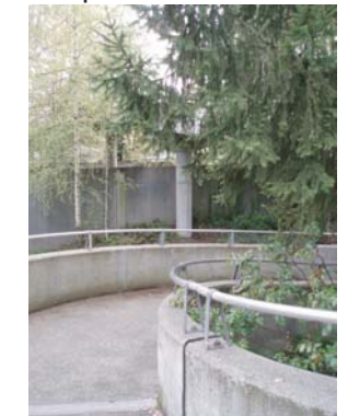
Encroaching vegetation on north access ramp
