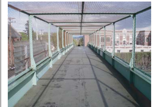
Although the bridge provides a 10' 6" curb-to-curb width, the extruded steel beams reduce the usable width to about 10'
