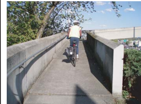
Although the bridge and access ramp width provides enough lateral clearance for one bicyclist, it may be difficult for multiple oncoming bicyclists to pass each other
