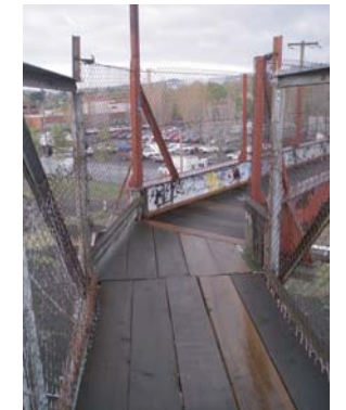
An alignment shift midway across the bridge creates two segments with differing widths
