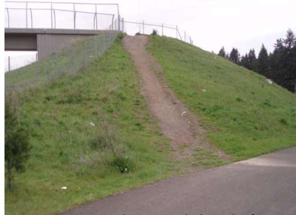
Figure 18 – Users have cut a hole in the fence to create a shorter access route to the I-5 at Main St. Bridge
