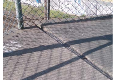
Expansion joint gap at east end of bridge structure
