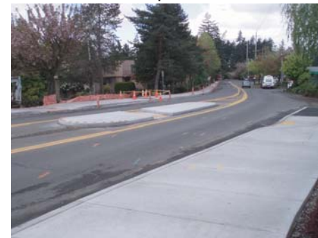
Mid-block pedestrian crossing under construction on SW Butner Road adjacent to bridge's south access ramp
