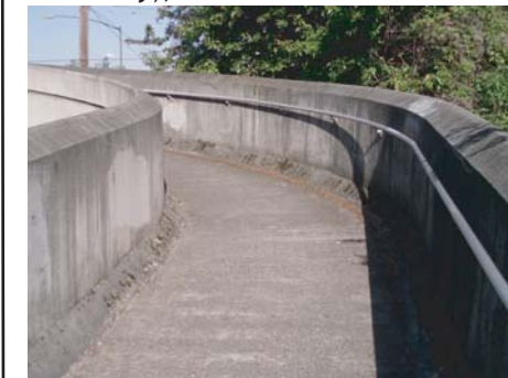
Railings are provided on one side of the bridge and access ramps
