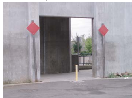
A smooth transition is provided at the base of the bridge's south access ramp with NE 142nd Ave.
