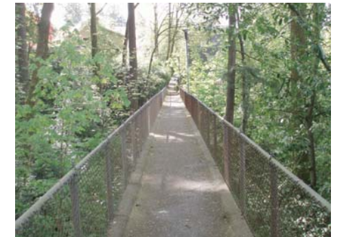
Extruded curbs reduce the bridge's usable width
