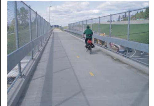
Bridge cross-section includes a 14' width (curbs and railings are flush with one another)
