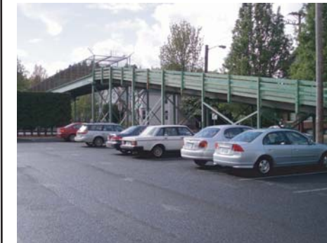
The east access ramp is fairly steep and lacks level landings
