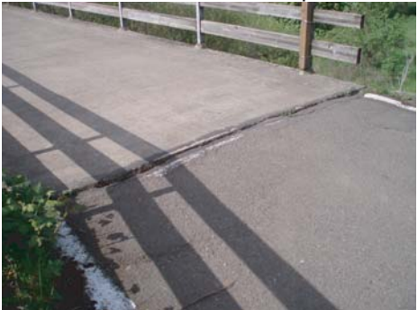
Pavement "lip" at bridge's north end
