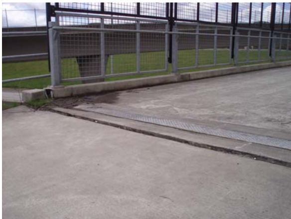
Figure 29 – Pavement “lip” at the I-5/Oregon 217 Interchange Bridge
