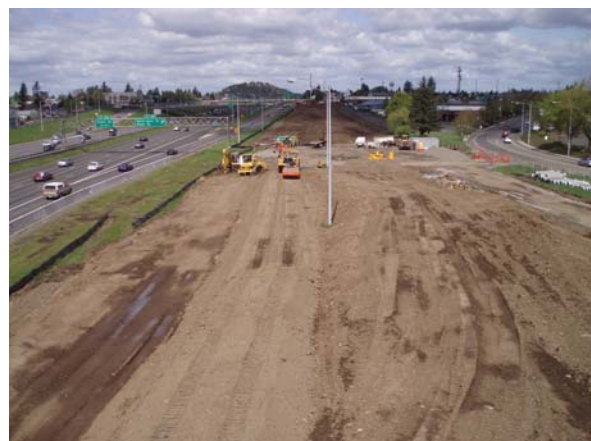
Figure 2 – Light rail station under construction near the I-205 at SE Main St. Bridge
