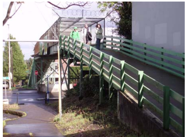
Figure 16 – Linear access ramps at the SW Hooker Street at Naito Pkwy. Bridge, and bus stop directly below the structure
