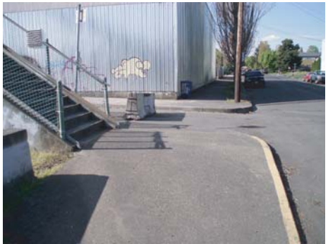
Curb ramps lacking where stairways meet surrounding sidewalks
