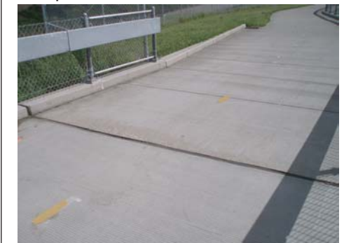
Minor expansion joint gap at bridge's west end
