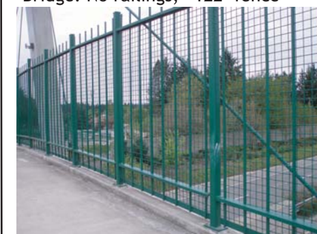
Railings not provided on bridge structure
