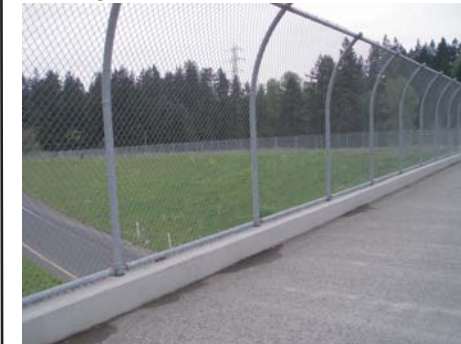
Railings not present on bridge structure
