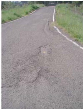
Rough pavement conditions on north access path
