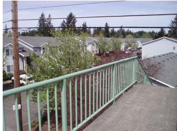
Figure 27 – Low-hanging electrical wires create safety issues at the SE Division St. at 136th Ave. Bridge
