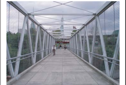
Bridge cross-section includes a 14' width (curbs and railings are flush with one another)
