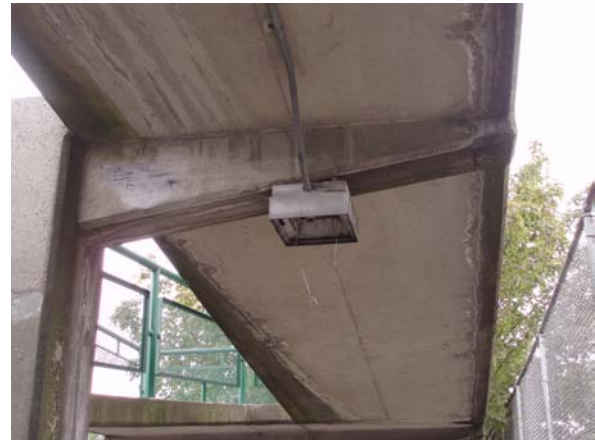
Figure 34 – Missing light at the N Columbia Blvd. at Midway Ave. Bridge
