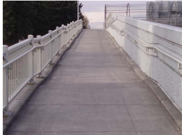
Figure 28 – Access ramp with level landings on the I-5 at N Failing St. Bridge
