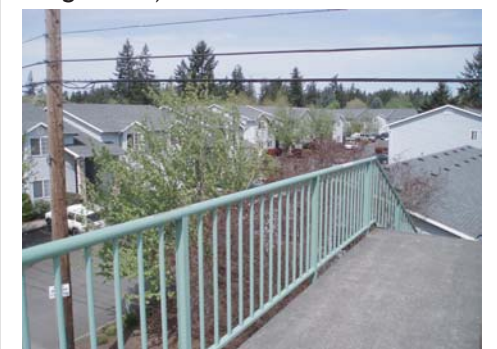
Low-hanging electrical wires above bridge
