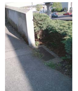
Drainage grate placed outside the bicycle/pedestrian travelway
