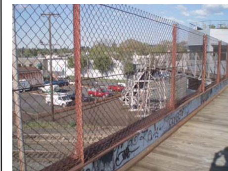
Railings not provided on bridge structure
