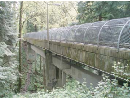
Lighting on bridge structure
