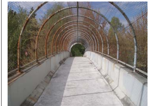
Extruded curbs reduce the bridge's usable width
