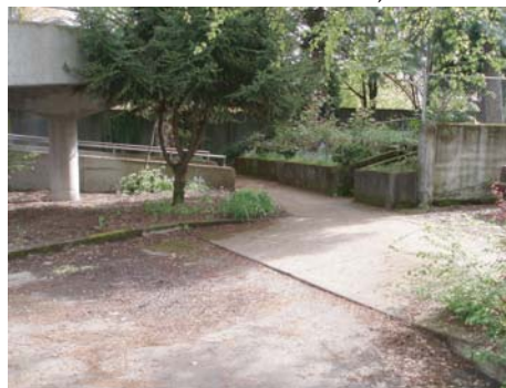
"Lip" on driveway apron at bridge's north access point
