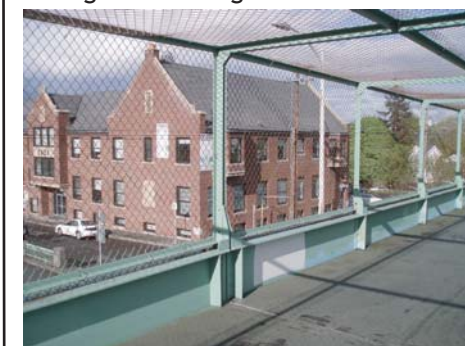
Railings are absent from the bridge structure
