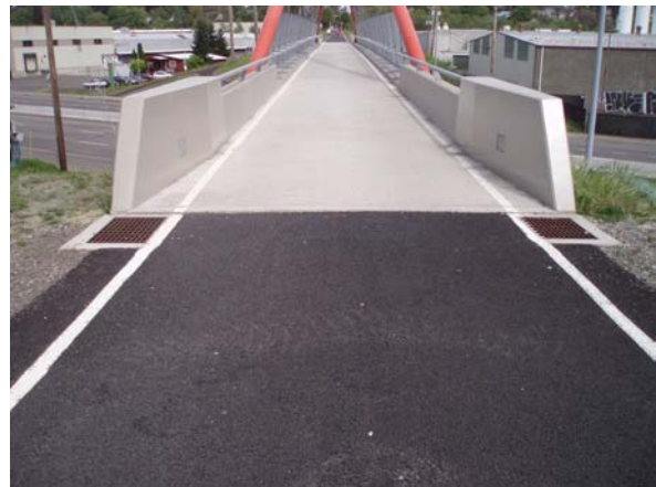
Figure 30 – Drainage grates placed outside the pedestrian/ bicycle travelway near the Springwater Trail at SE McLoughlin Blvd. Bridge
