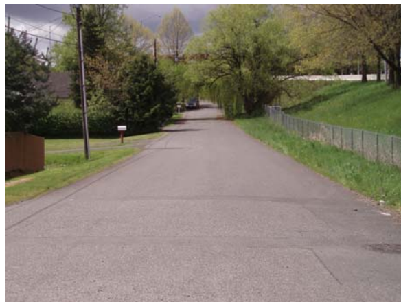
Figure 8 – Many streets near the I-5 at Barbur Transit Center Bridge lack sidewalks
