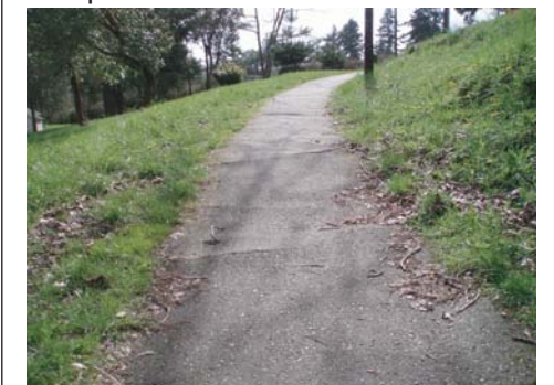
Pavement cracking/heaving on east access path
