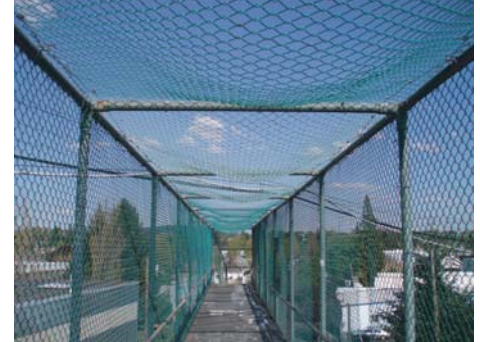
Sinking overhead fence on bridge structure
