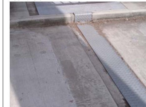
Expansion joint gap at bridge's south end
