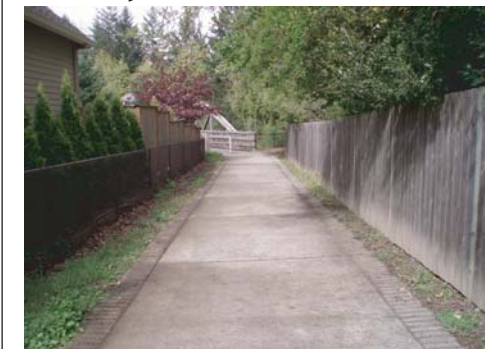
Minor vegetation encroachment on east accessway
