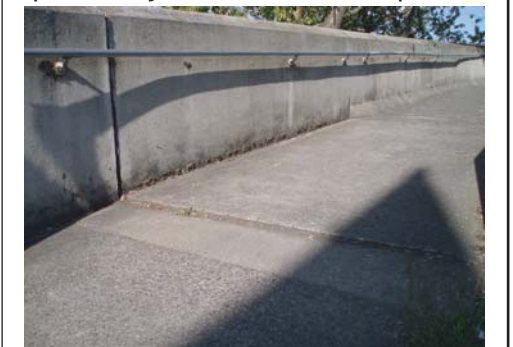
"Lip" on north access ramp could pose difficulties for "wheel users"
