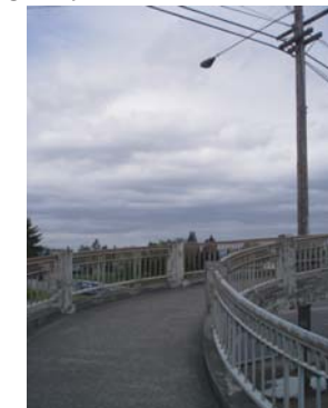
Light poles on N. Lombard St. are the bridge's primary illumination source
