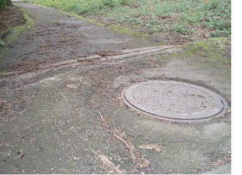
Poor pavement conditions on north path
