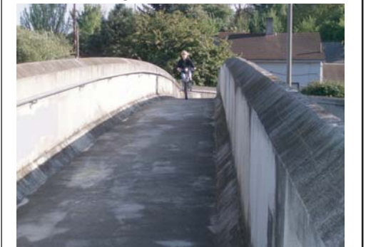
Extruded curbs reduce the bridge's usable width
