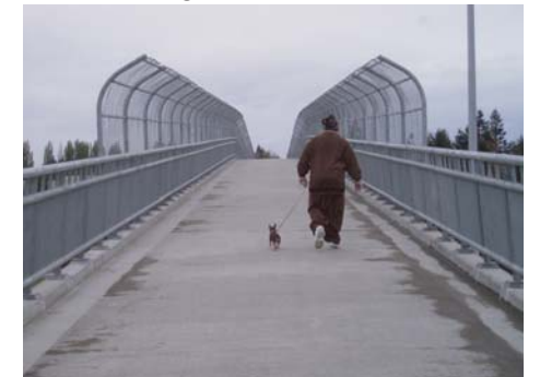
Bridge cross-section includes a 14' width (curbs and railings are flush with one another)
