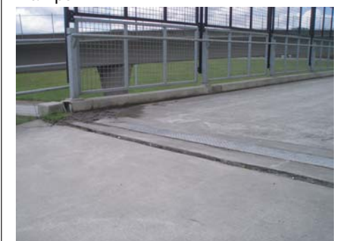
Pavement "lip" at bridge's east end
