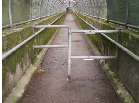
Figure 25 – Horizontal railings create a tight “pinch point” at both ends of the Trillium Cr. Bridge
