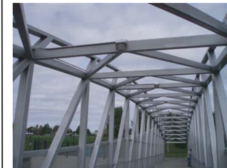
Overhead lighting on bridge
