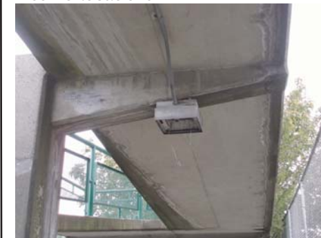
Missing light on south side of bridge
