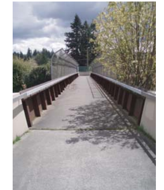
Vegetation encroaching on bridge structure
