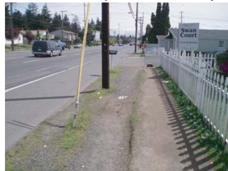
Sidewalk gap on SE Division St. immediately east of the bridge
