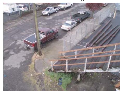
Curb ramp in poor condition at bottom of west stairway
