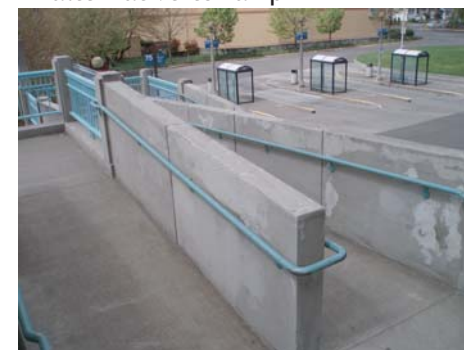
Narrow access ramp with multiple switchbacks complicates bicycle access on the bridge's north end
