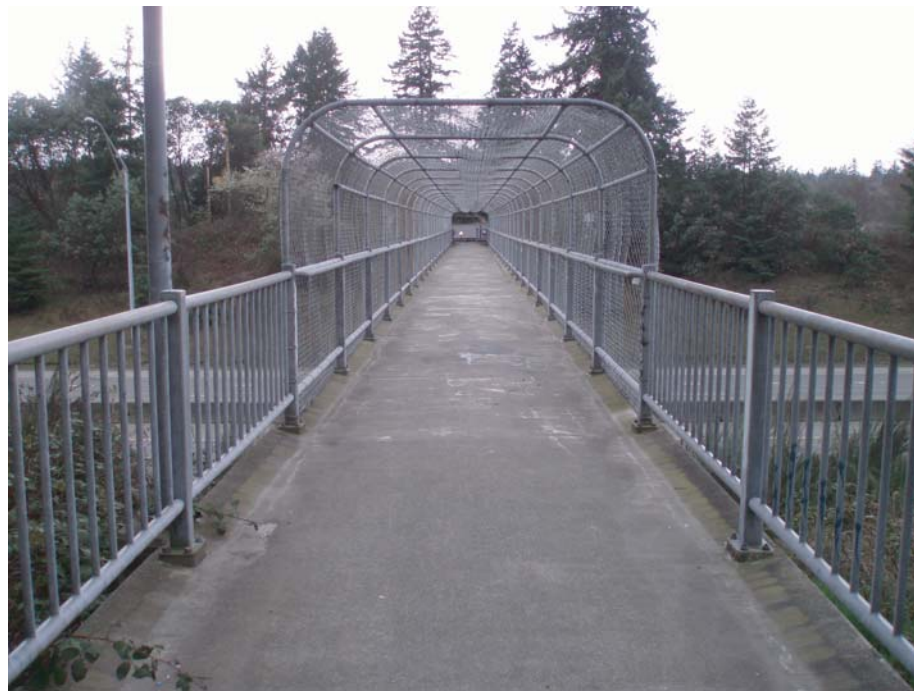
Location: Bremerton, WA
