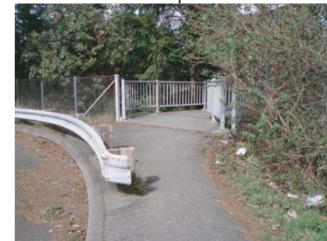
The lack of curb ramps complicates bridge access for some users
