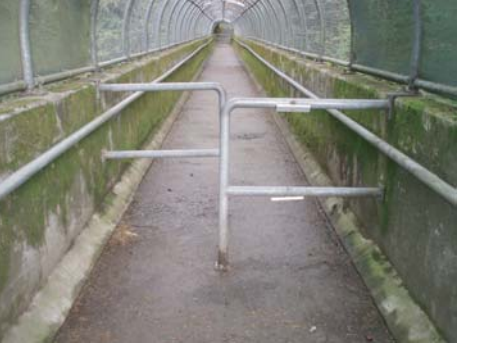
Railings obstructing travel on the bridge
