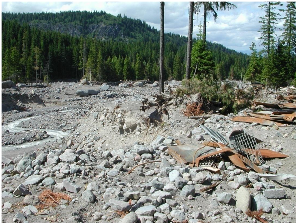
Figure 12. Damaged water intake structure for Hood River Irrigation District on Eliot Creek.
