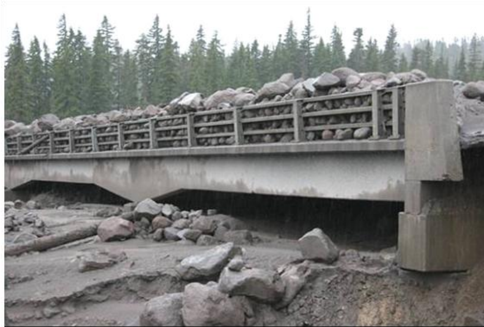
Figure 25. White River Bridge covered by debris flow deposit (ODOT photo)
