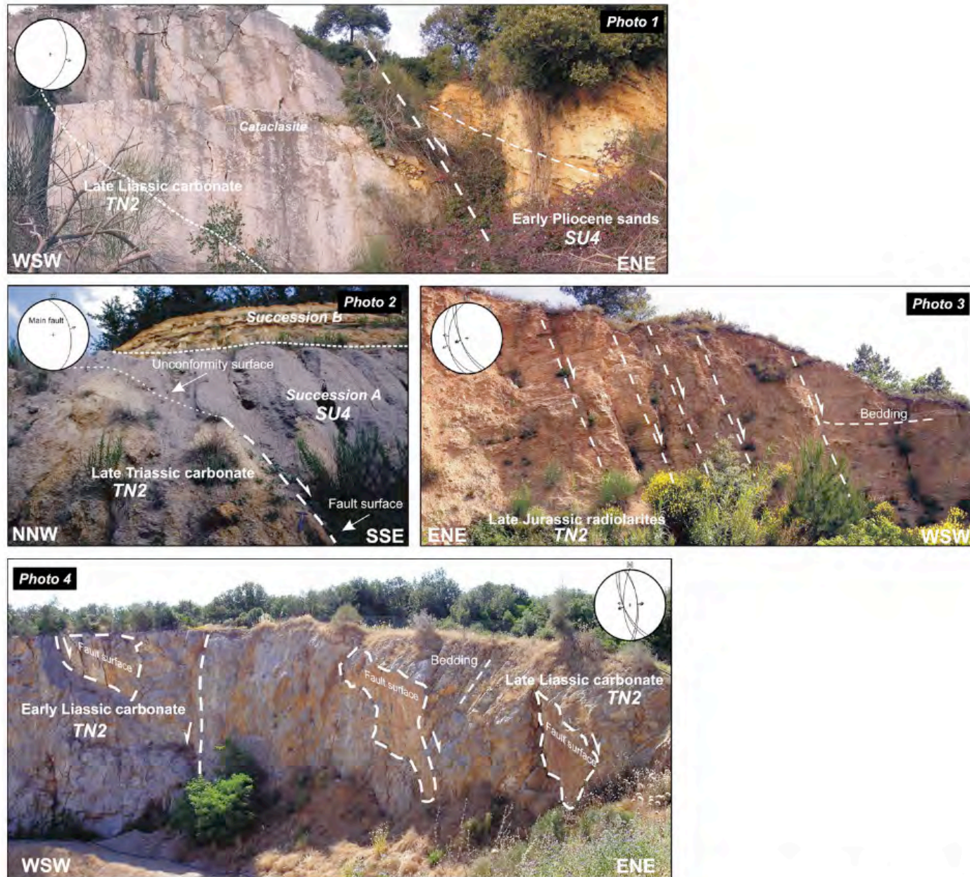
Fig. 10. Minor faults associated to the Rapolano Fault exposed in different outcrops indicated in the Fig. 9. Photo 1 illustrates a normal fault separating Early Pliocene sands and clayey-sands from the Late Jurassic carbonate (Calcare selcifero Fm) of the Tuscan Nappe. Photo 2 shows a sin-sedimentary normal faults active during the deposition of the succession A (Early–Middle Pliocene lignite bearing clay and silt); The Succession B (Middle Pliocene sands) buried the fault constraining its age (see the text for more information). Photo 3 illustrates parallel normal faults affecting Jurassic radiolarites (Diaspri Fm) of the Tuscan Nappe; Photo 4 shows some normal faults affecting Jurassic carbonates (Calcare massiccio Fm) of the Tuscan Nappe.
