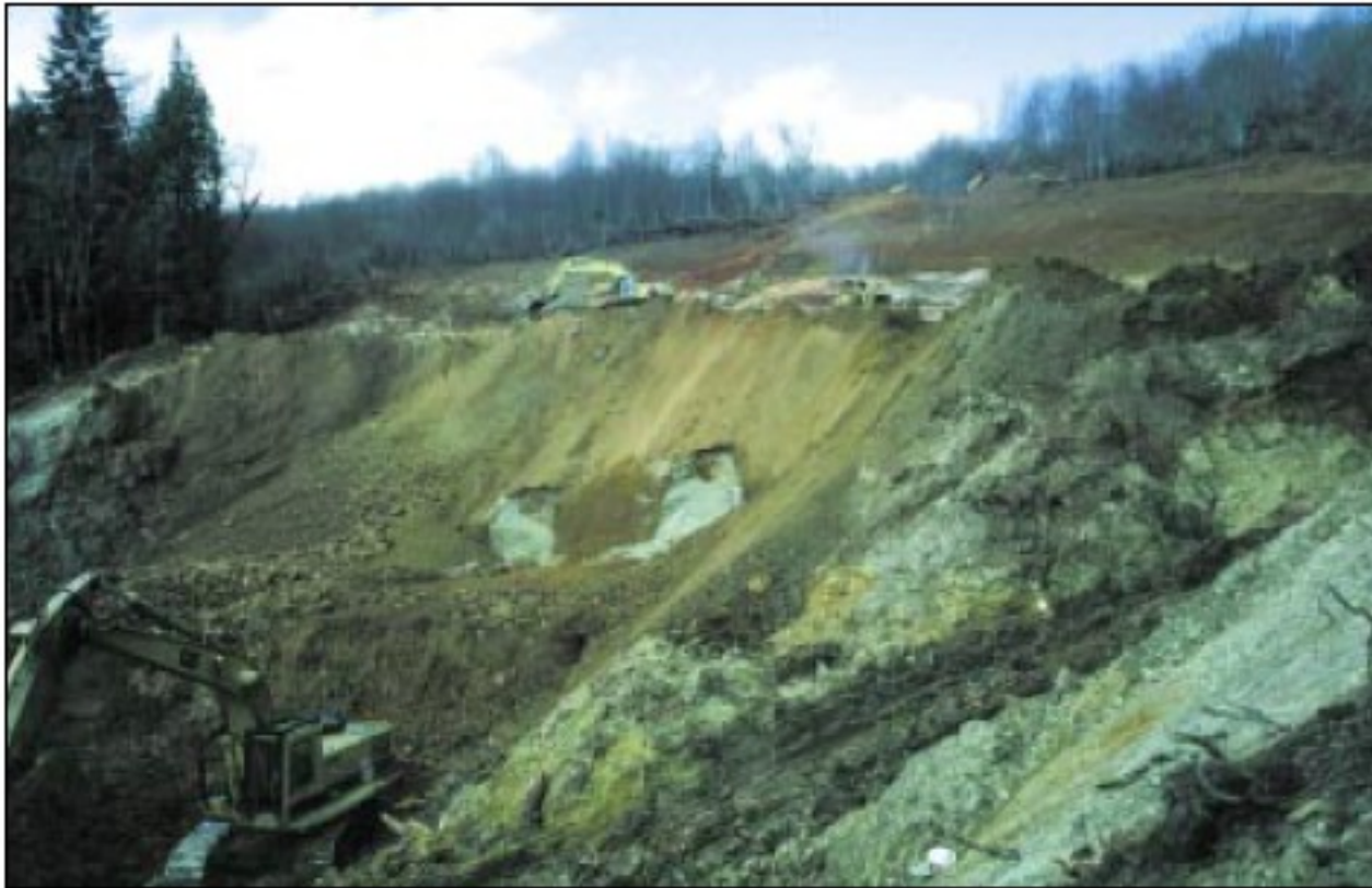
Figure 10 Head-scar area of slump-debris flow shown in figure 9
