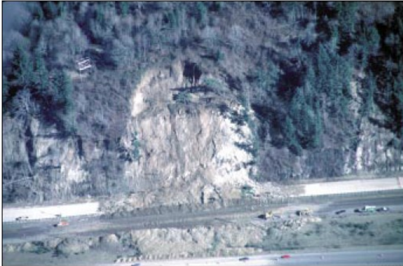
Figure 18. Slump north of Woodland, Washington that covered I-5 and the Burlington Northern-Santa Fe rail line.
