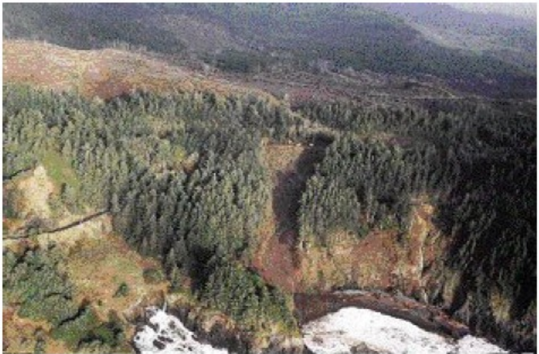
Figure 10. Cape Foulweather landslide. The downslope lanes of coastal US Highway 101 was damaged from a fill slope failure in December 1999. Repair work lasted about one month. (ODOI 33 photo)
